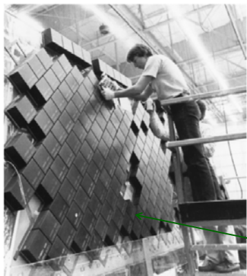
FIGURE 23.17 Photograph showing the installation of thermal protection ceramic tiles on the Space Shuttle Orbiter.
