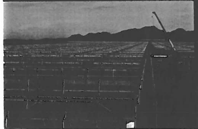
Crews work around the clock installing mirrored parabolic trough collectors — built on site — that will cover 3 square miles at Abengoa's Solana Plant in Ariz. Credit: Dennis Schroeder, NREL
