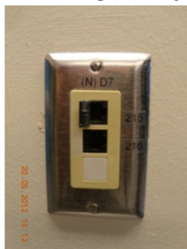
Figure 5: ENCS internet hub D7 with Ethernet jacks no. 215 and 216
